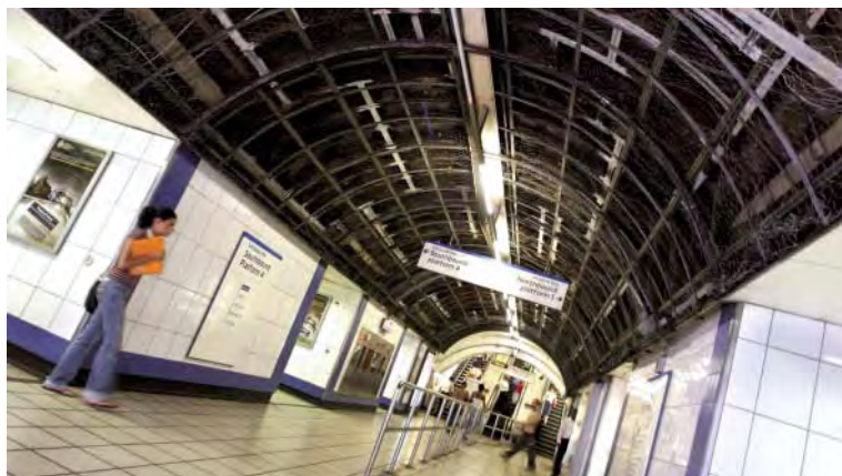
An innovative system at Victoria should cool things down a bit this summer.
